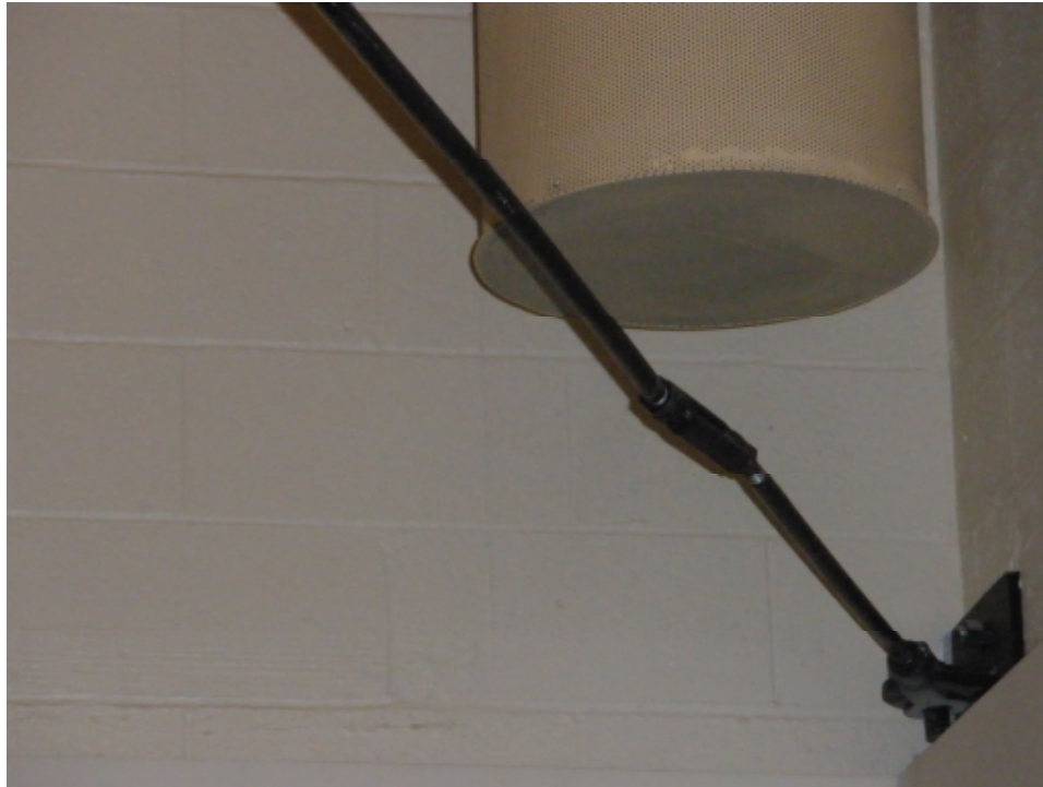
Photo 6: Kink in diagonal bracing rod at Library.
