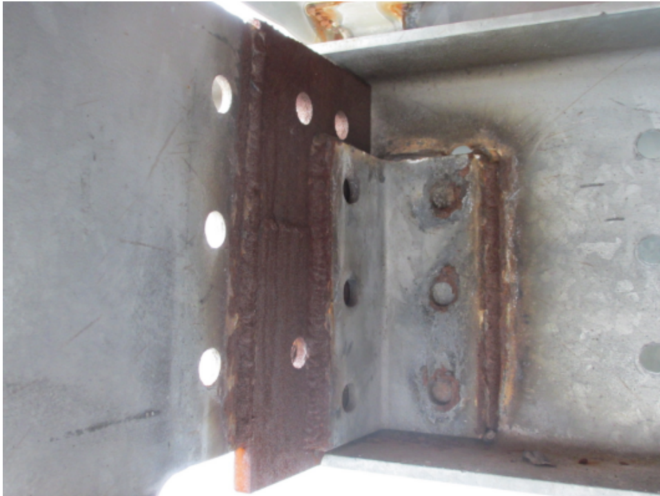
Photo 2: Fabrication/MEP coordination error at AHU-4 RTU frame.
