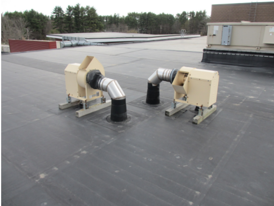
Photo 8: Typical rooftop LEF installations, unsecured, on wood sleepers.
