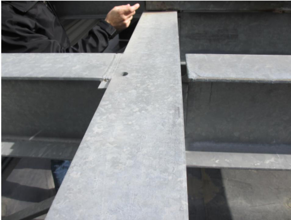
Photo 10: Dunnage frame at AHU-1, cantilevered screen is to the left. Note moment connection (welded top flange) is provided for the beam coming in from the left, but is not provided on the beam to the right.
