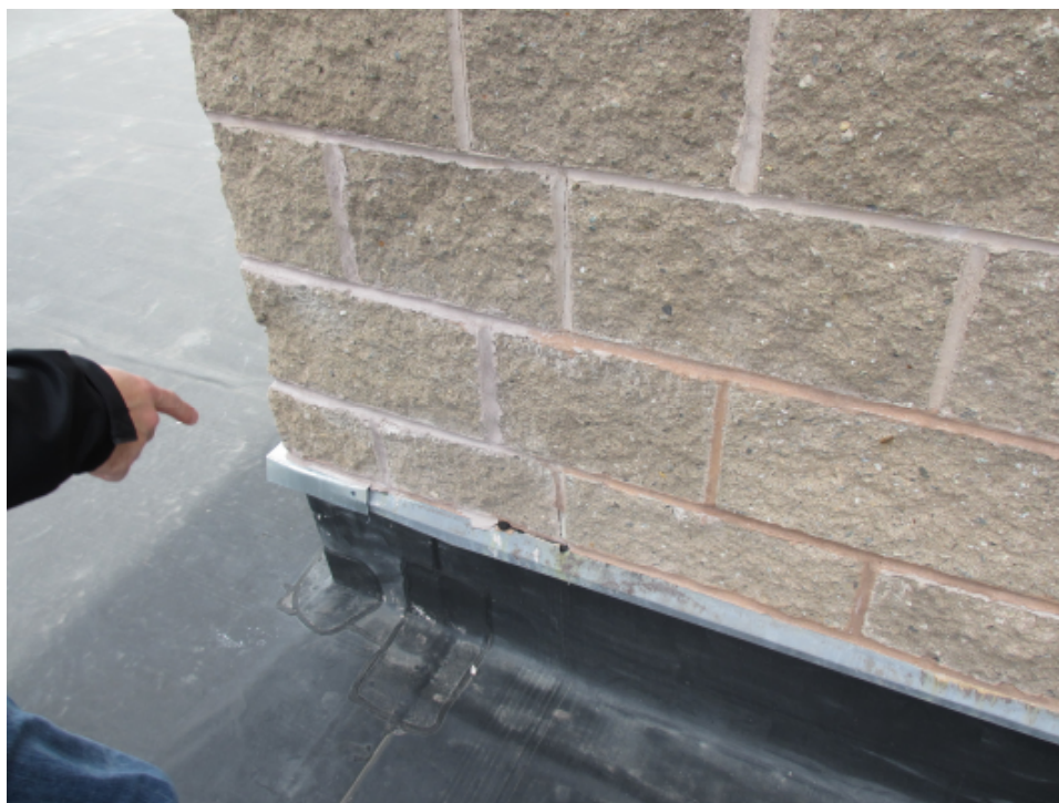
Photo 14: Exterior wall at SE corner of auditorium: CMU veneer has been re-pointed at least twice. This is likely indicative of a wall cavity drainage issue at this corner.
