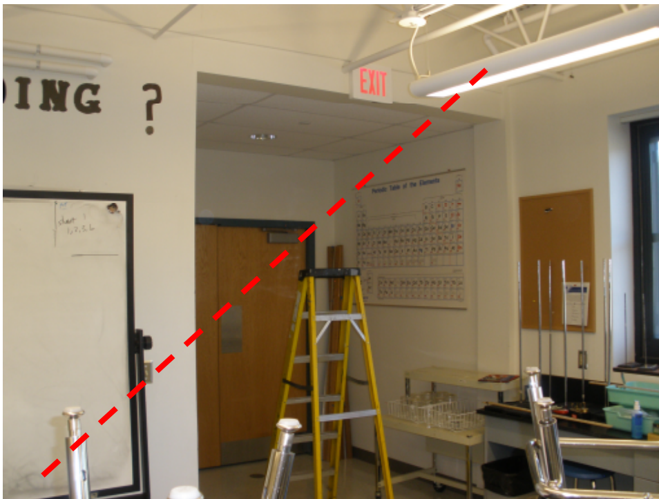
Photo 5: Science lab: Diagonal brace at alcove not per construction drawings (relocation of brace was approved by the SER during construction).
