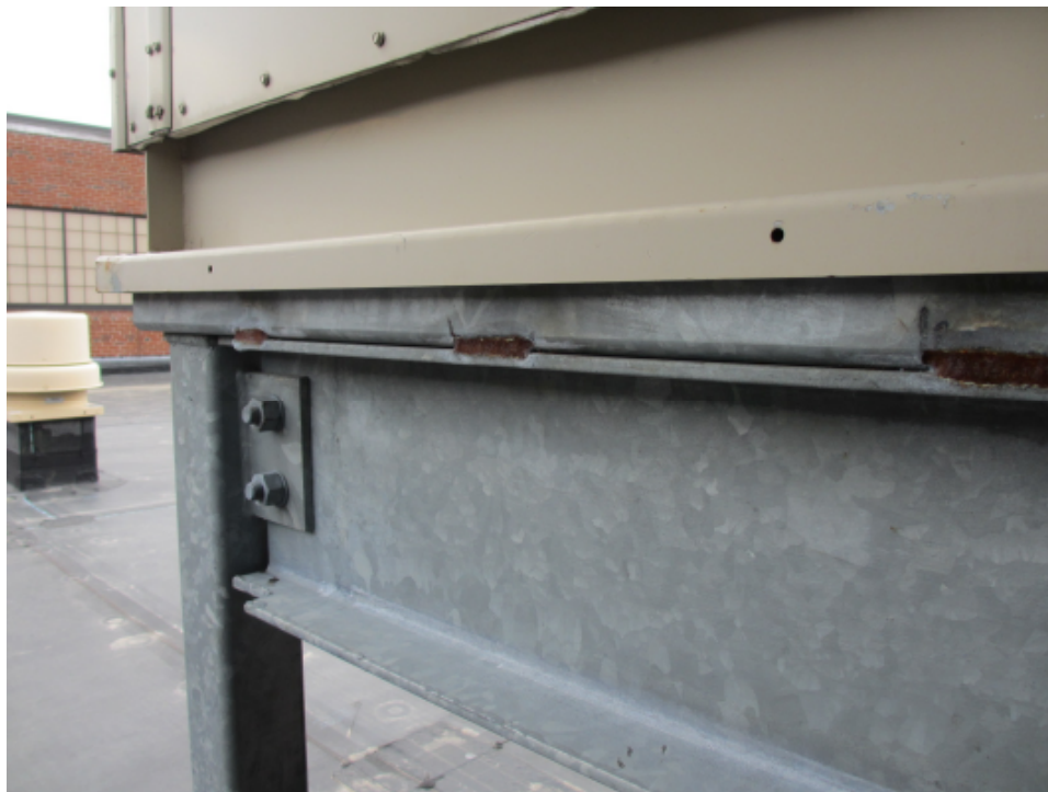
Photo 13: Welds on AHU frames should be treated with zinc rich paint to retard corrosion.
