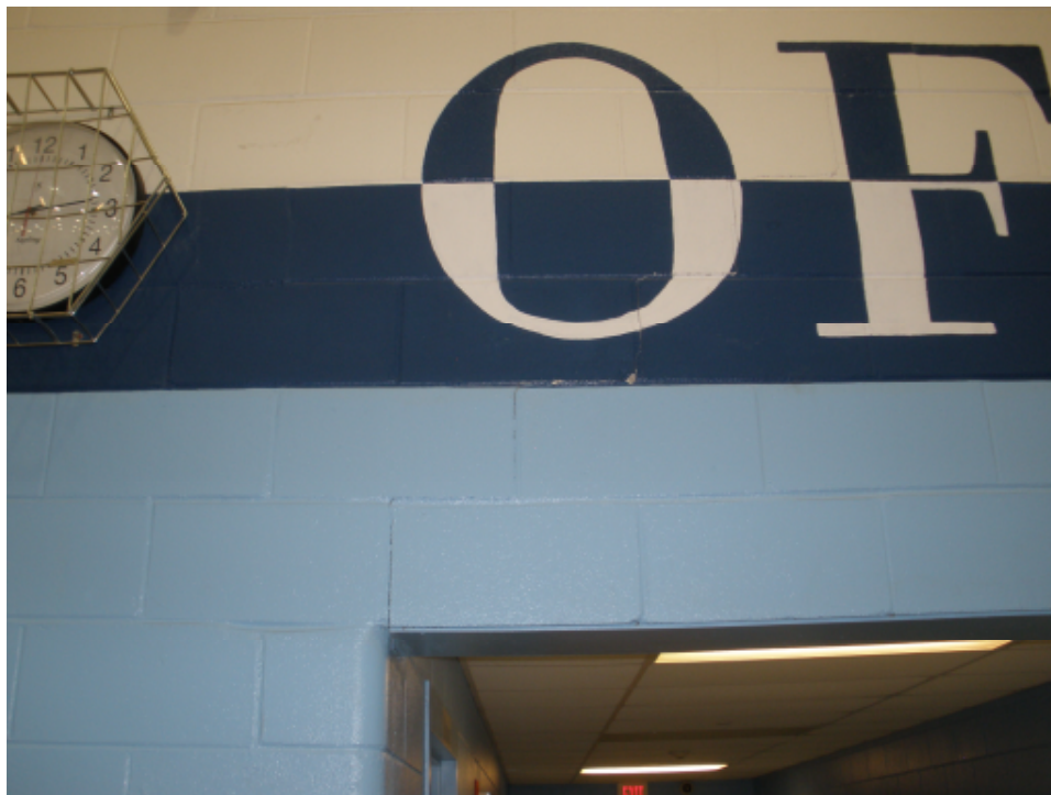
Photo 3: Step crack over central entry portal in S wall of gym.
