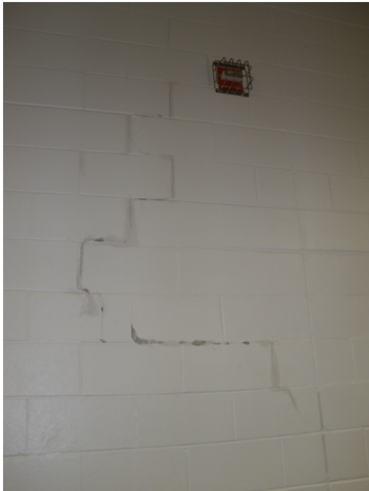
Photo 1: Interior north wall of gymnasium at gym centerline: Step crack near fire beacon, above bleachers, does not follow the vertical control joint. (Control joint is visible at bottom right corner of this photo.)
