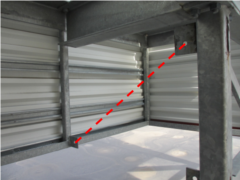
Photo 12: AHU-1 rooftop frame – note missing bracing angle.
