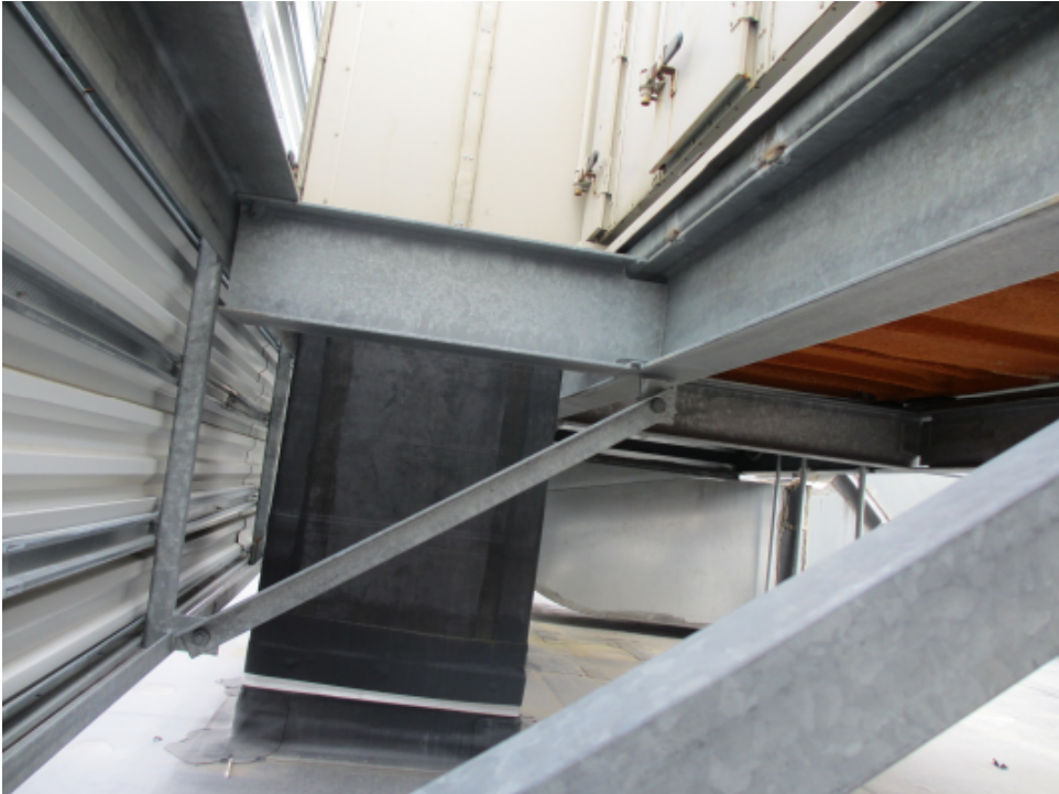
Photo 11: AHU-1 rooftop frame – note bracing angle to bottom of screen.
