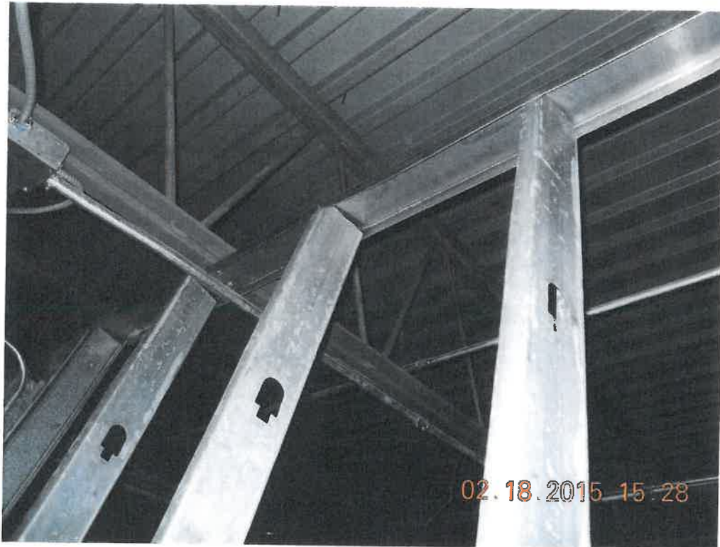
Metal stud wall allows for no movement of roof joists.
