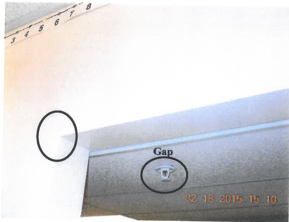
Drywall stress crack
