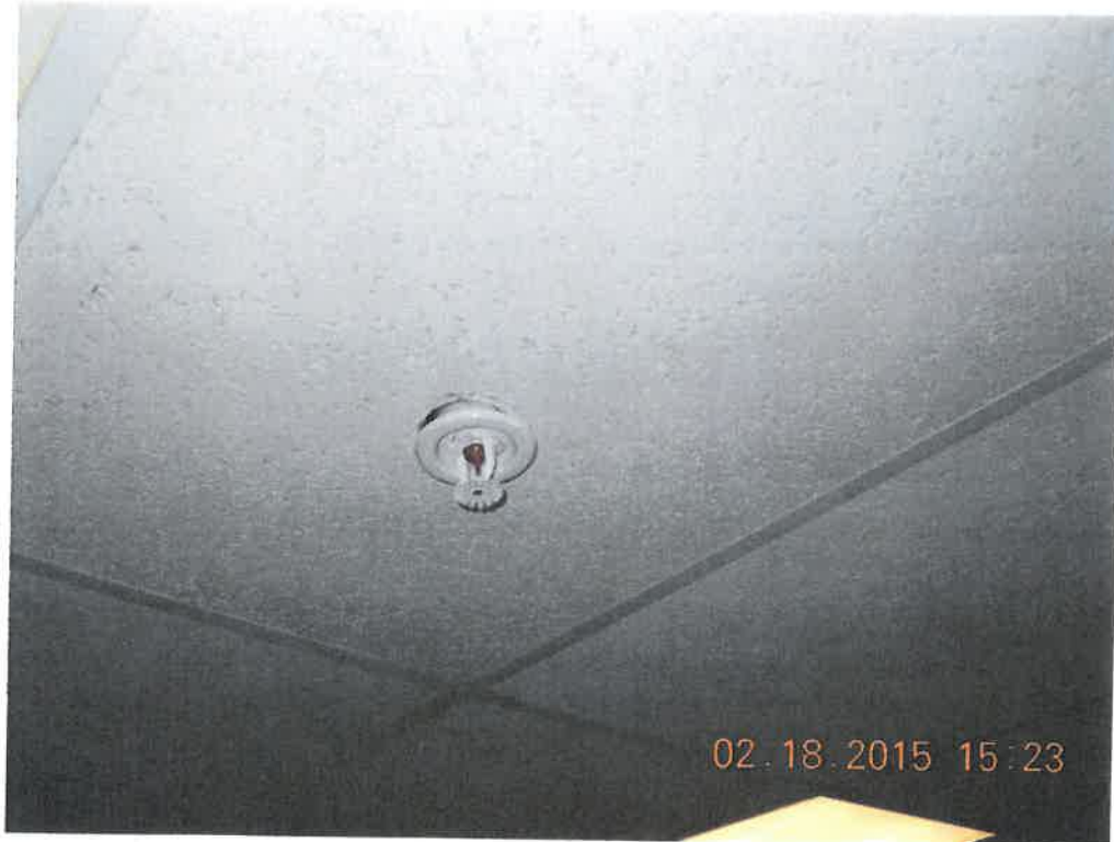
Sprinkler head moves downward as roof joists deflect downward.
