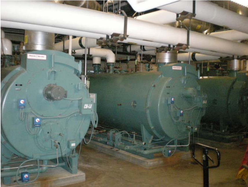
Heating Plant – Three Fire Tube Boilers (2004 Installation)
