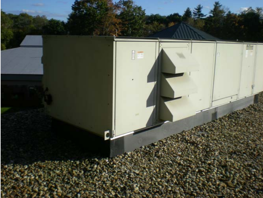
Multi-Purpose Room Roof Top Ventilation Unit (1989 Installation)
