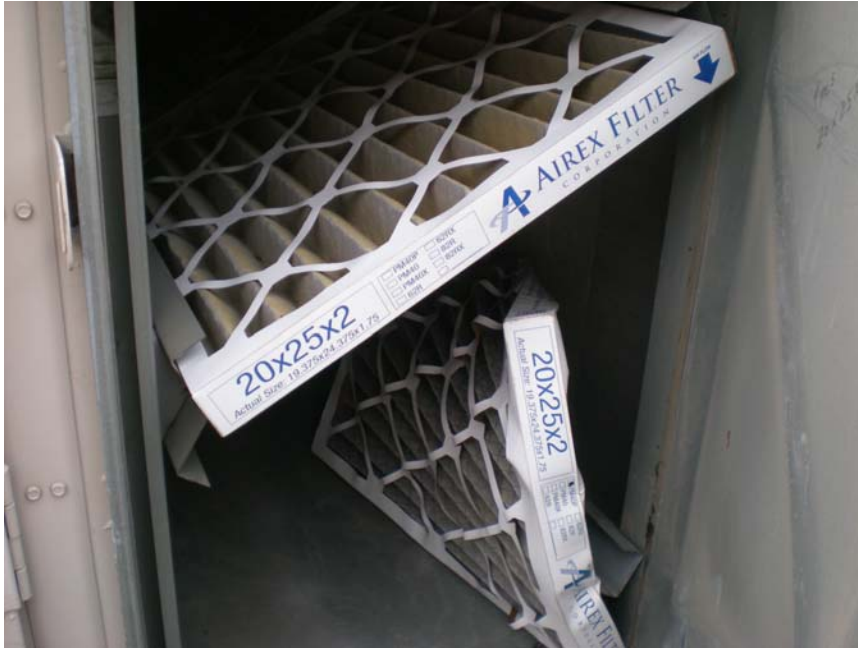
Crushed, dirty filters at Industrial Arts Air Handler (AHU-9)
