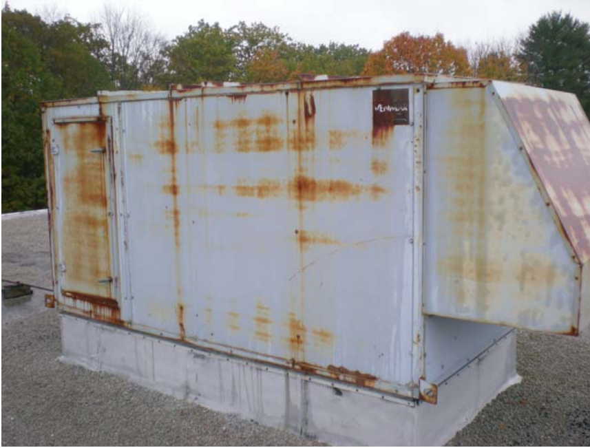
Typical Energy Recovery Ventilation Unit (1995 Installation)
