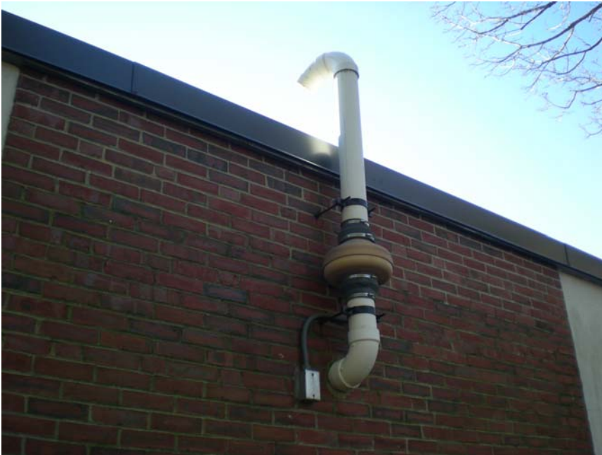
Typical Radon Vent System at North Wing – Fan Powered
