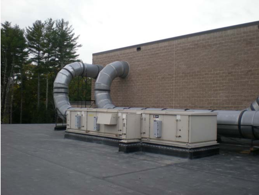
Typical Rooftop Air Handling Unit and exposed ductwork (2004 Installation)
