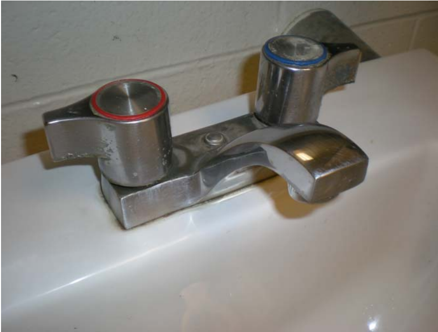
Typical lavatory faucet
