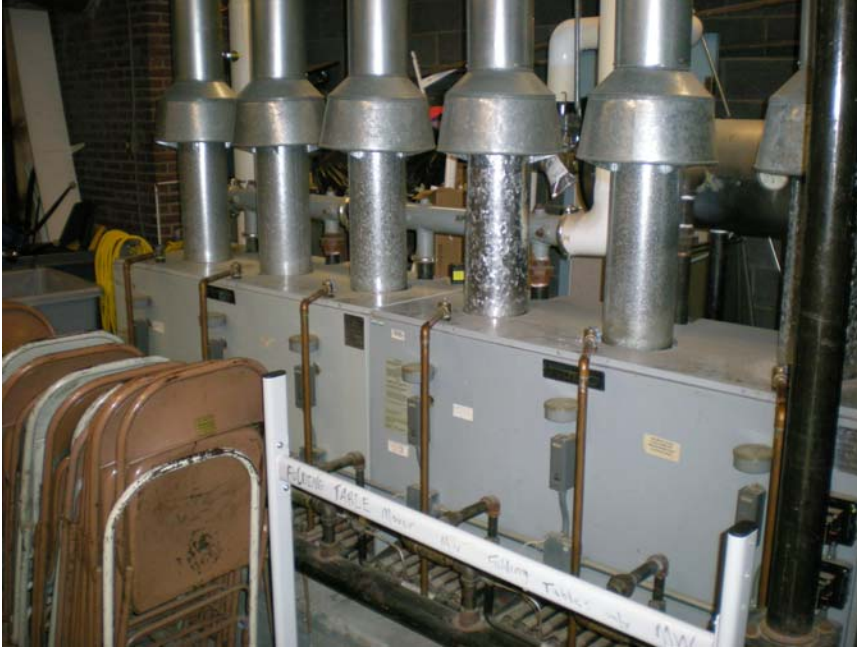
Modular Cast Iron Boilers with atmospheric burners (1991 Date of Manufacture)
